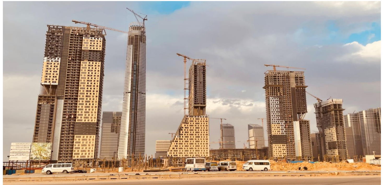
Egypt's New Administrative Capital about 45 km east of Cairo. Photo: Ulla Huotari
